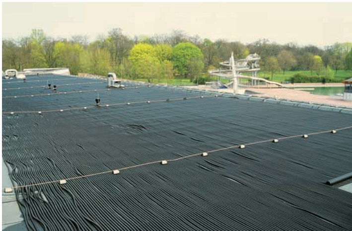
Figure 16: Solar thermal system for swimming pool heating in Pankow, Berlin (source: DGS)
