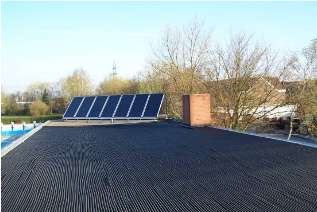
Figure 6: Absorber- and flat-plate collectors for solar heating
