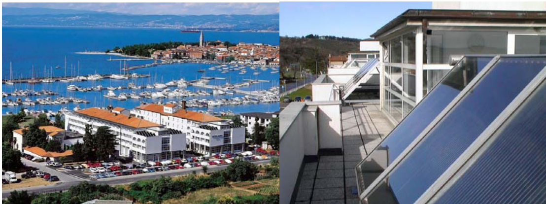
Figure 1: Flat Plate Collectors in Hotel Delfin (Source: www.solarge.org)
